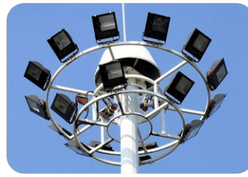
HIGH MAST LIGHT
